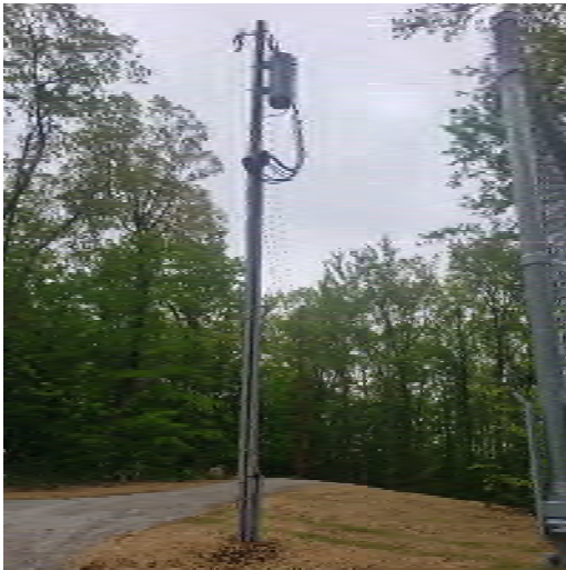
Utility pole and transformer
