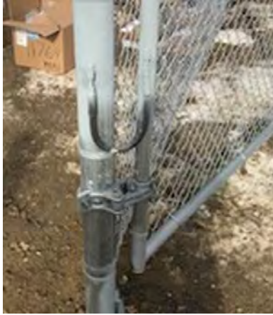
Fence gate grounding
