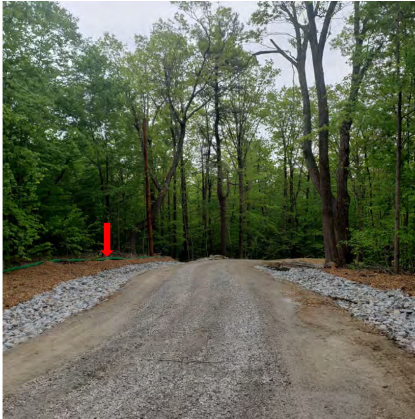
Monterey, MA – Gravel Driveway with Perimeter Erosion Control Log
