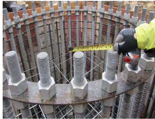
Monopole anchor bolts
