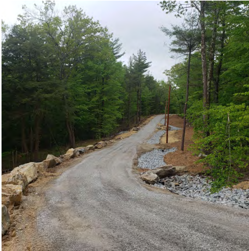
Monterey, MA – Gravel Driveway with Boulder Protection Barrier
