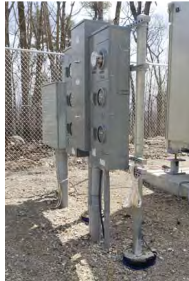
Meter bank front
