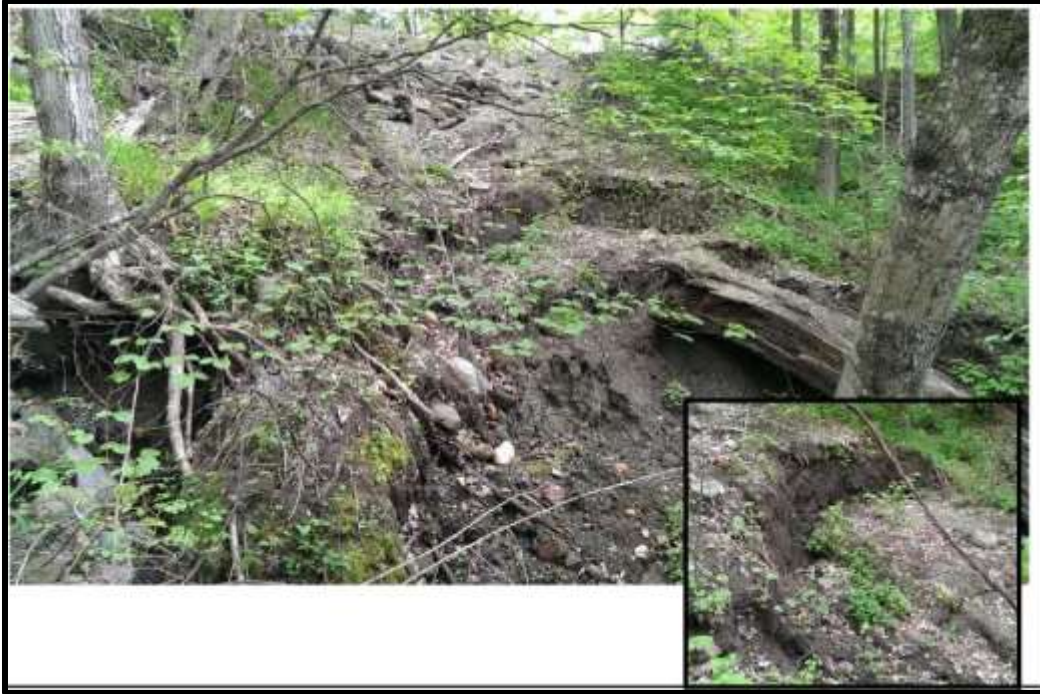
Midslope below northern erosion area. Headscarp from recent slope failure in foreground. Riprap emergency repair (2016) in background. Leaning and undercut trees visible. Close-up of headscarp shown in inset.
