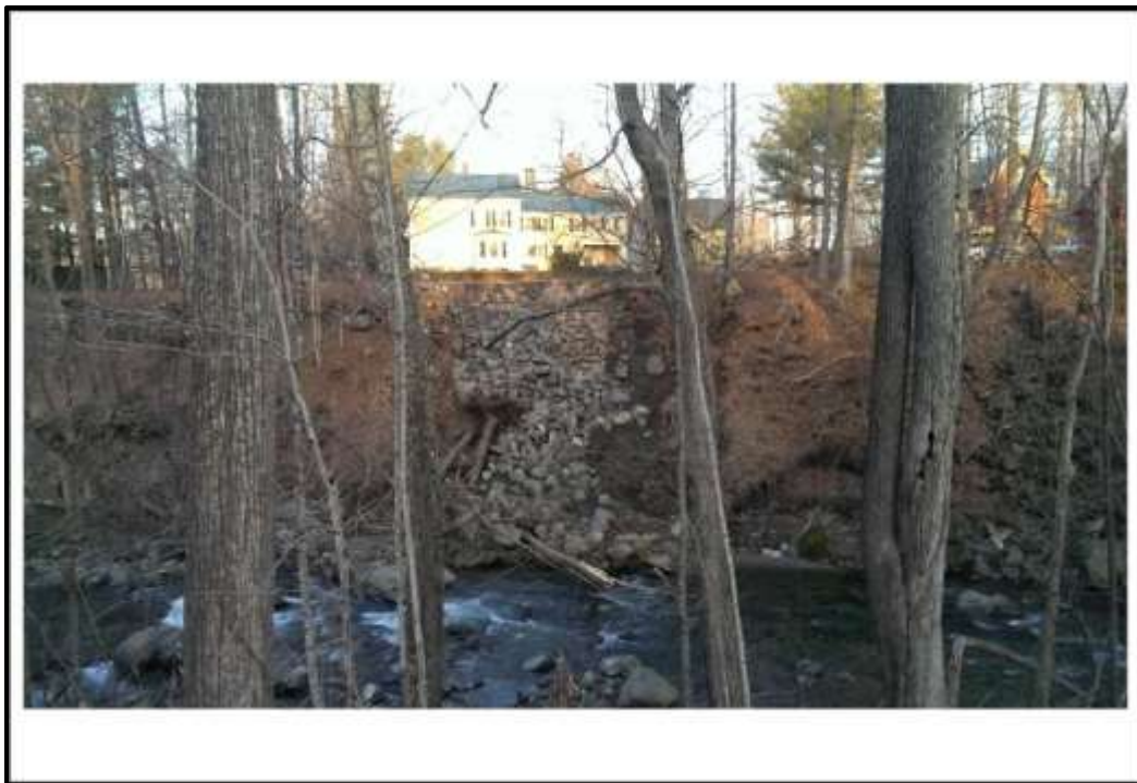
View of southern erosion area from Route 116 (across river). Source: Conway HMGP Application.
