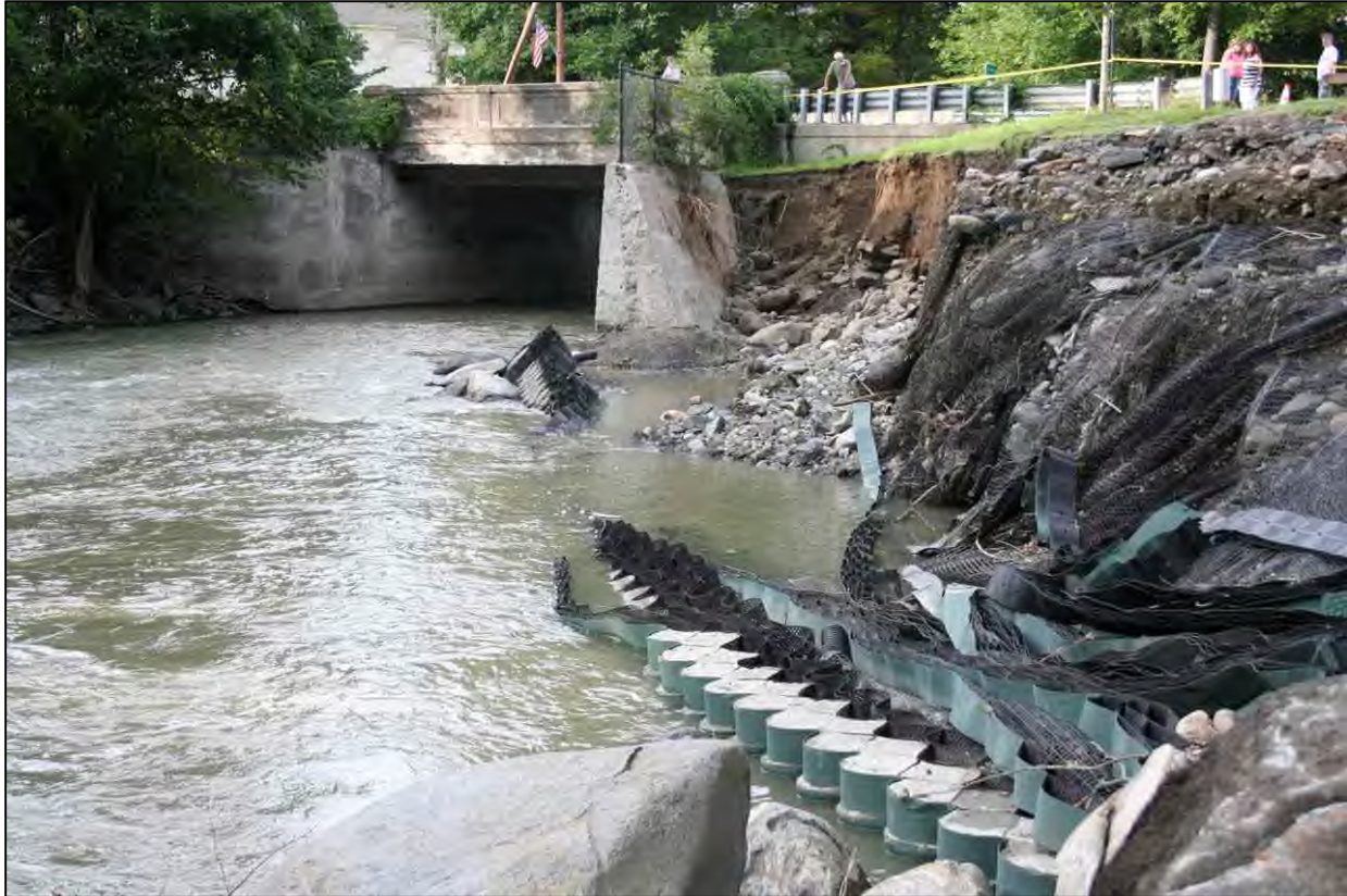
Damaged gabion retaining wall below the Route 116 Bridge along the South River, after Tropical Storm Irene in 2011
