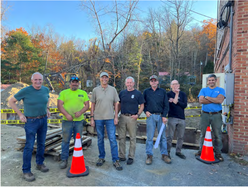
The crew working on the beginnings of the new Public Safety Building offices: Left to right are Dave Vreeland, Ben Hay, Peter Jeswald, Ken Ouimette, Ron Sweet, Walter Goodridge and Chris Herrmann.
