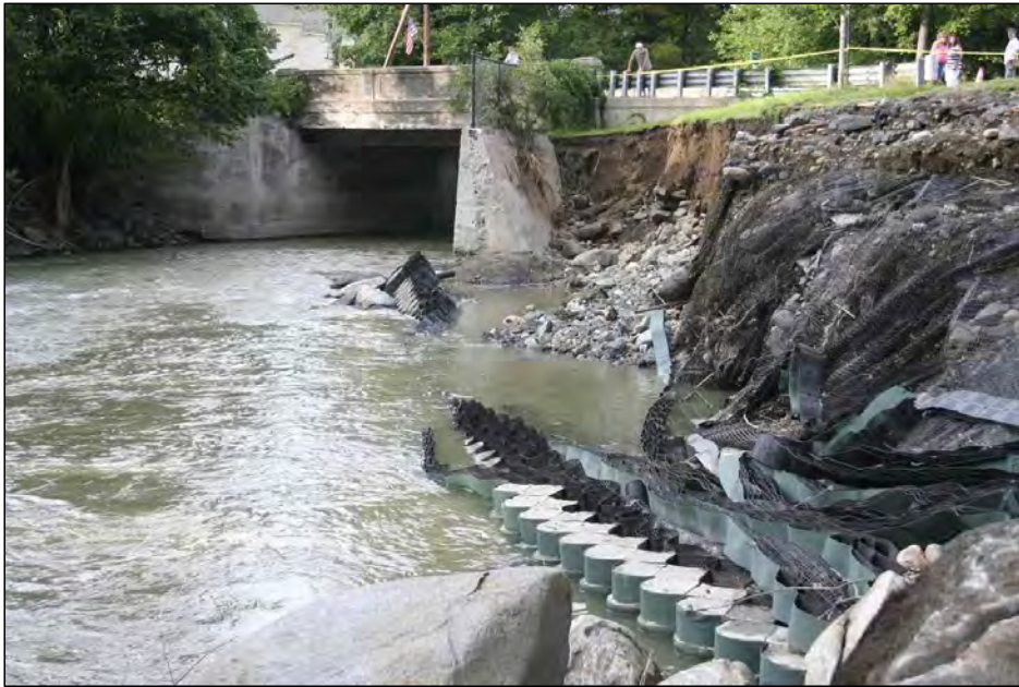
Damaged gabion retaining wall below the Route 116 Bridge along the South River, after Tropical Storm Irene in 2011 ( image credit? )
